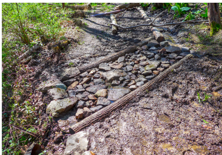
Trail structures such as open culverts are devices that help keep trails passable.
