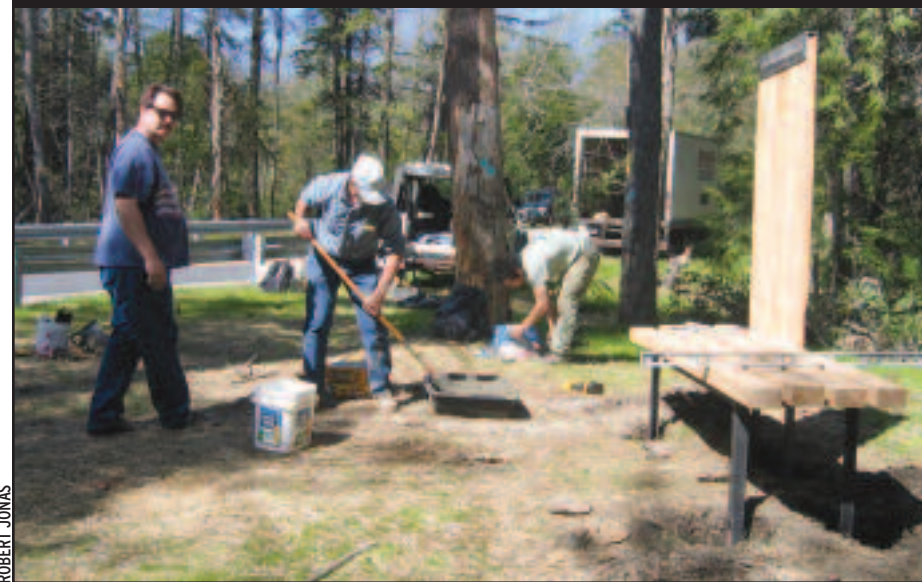
Volunteers Eric and Ron Luna and project manager Chris Ingui install a trail kiosk with bench in West Milford.
