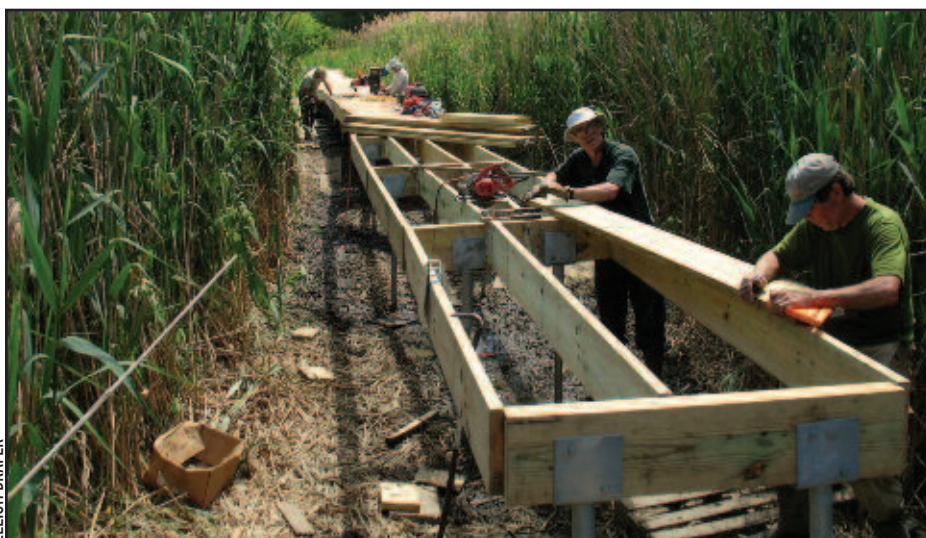
Volunteers with the Appalachian Trail Dutchess-Putnam Committee continued work this spring and summer on the big boardwalk project over the Great Swamp in Pawling, NY.
